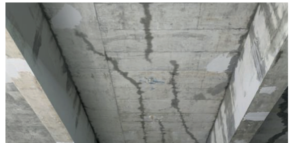
Typical cracking parallel to beam (90%)
