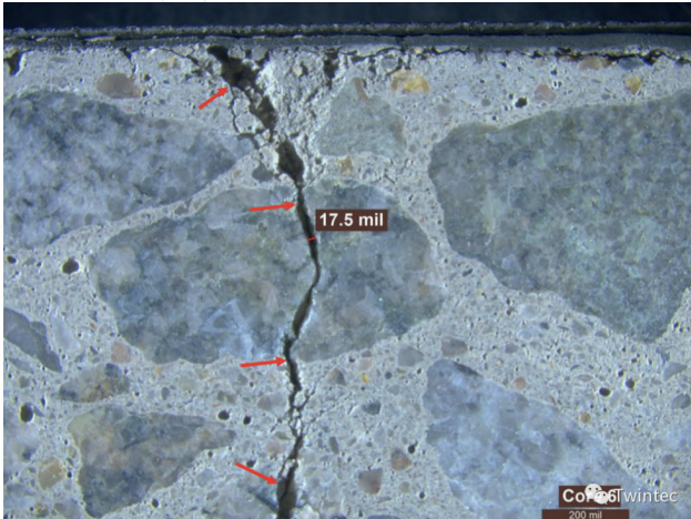
Figure 9. Core 6. Close-up image of the top surface region. The measurement near the center of the image indicates typical crack width along the lapped surface within the top region. Red arrows indicate cracking, which extends the full depth of the sample. The crack propagates through two coarse aggregate particles in this region.
